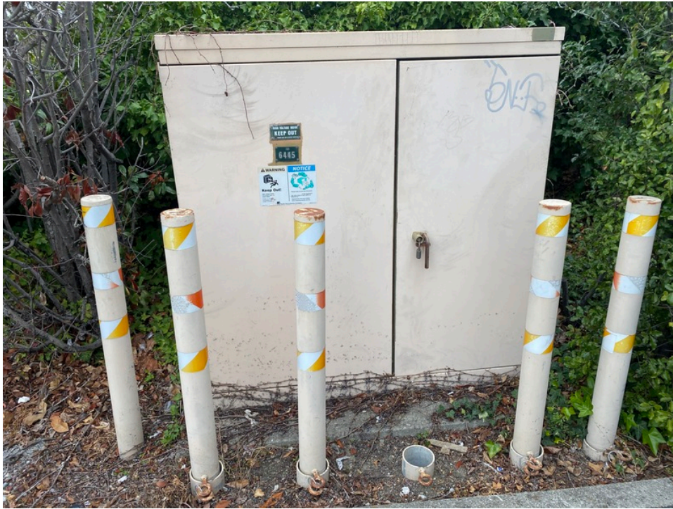
29. On-site pad-mounted transformer
