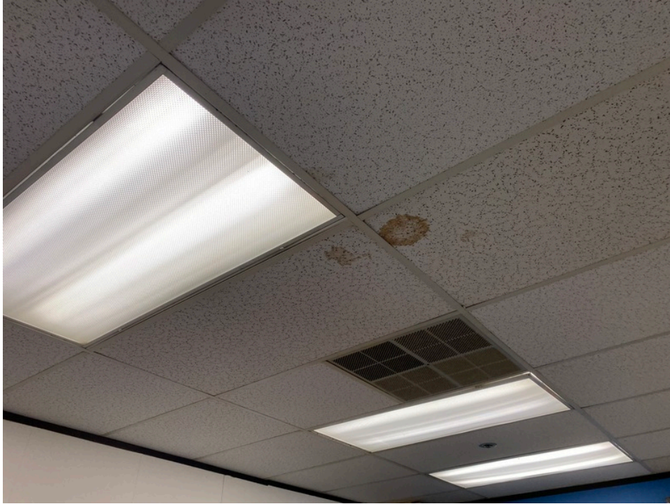
27. Observed water-stained ceiling tiles
