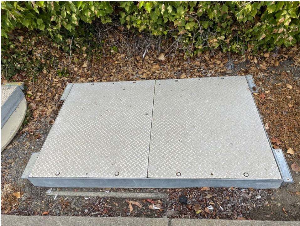
30. On-site transformer vault
