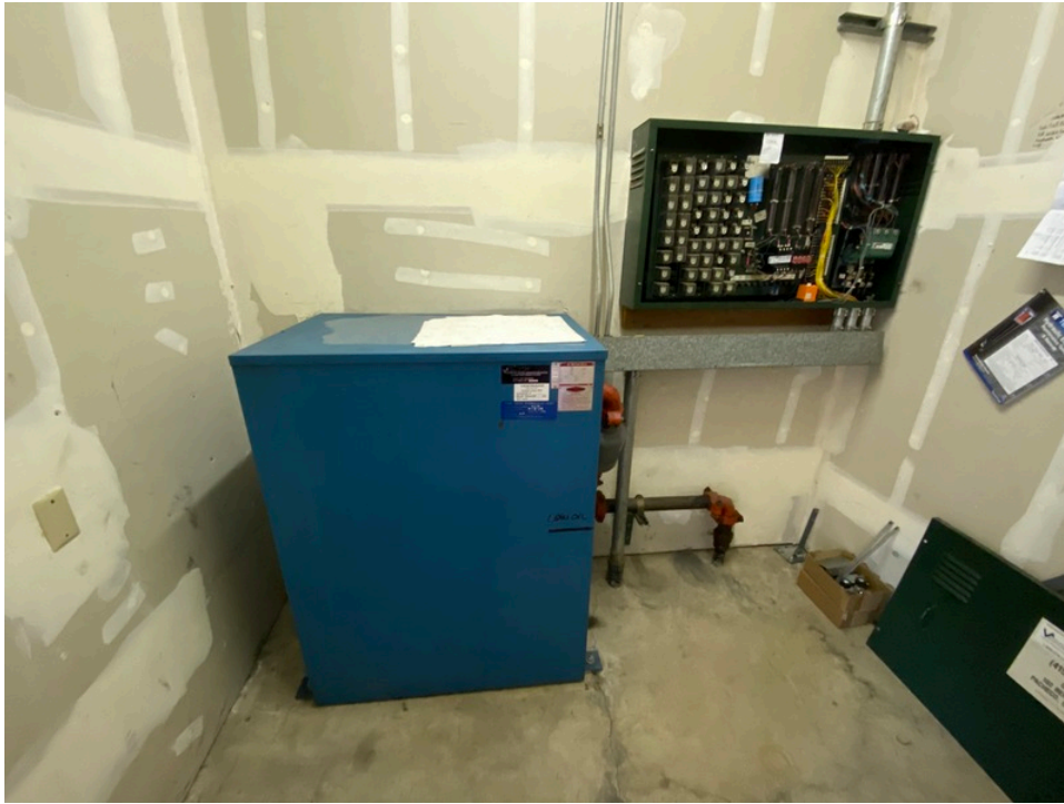
25. Elevator equipment room
