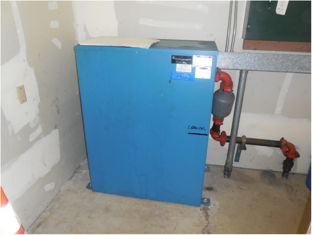
10 Subject Site Hydraulic elevator equipment.
