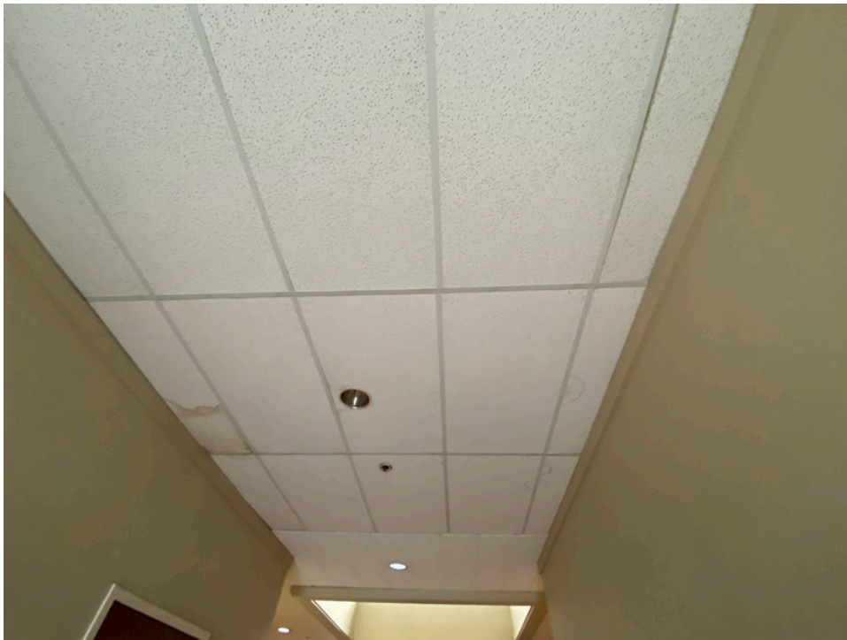
28. Observed water-stained ceiling tiles
